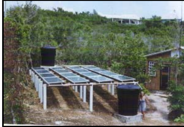
A Large Solar Distiller Array!
